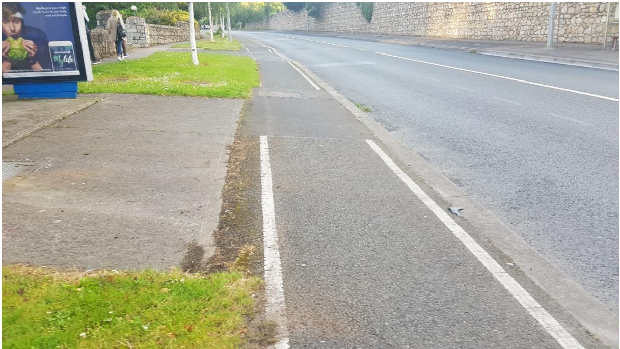
Figure 29: Layout at Bus Stop on Brewery Rd, N31 (Note No kassel kerbs)
