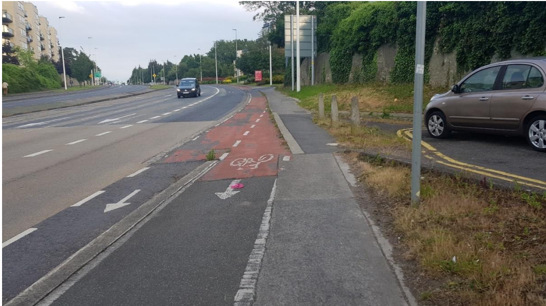
Figure 20: Trip hazards and poor surfacing within VRU facilities
