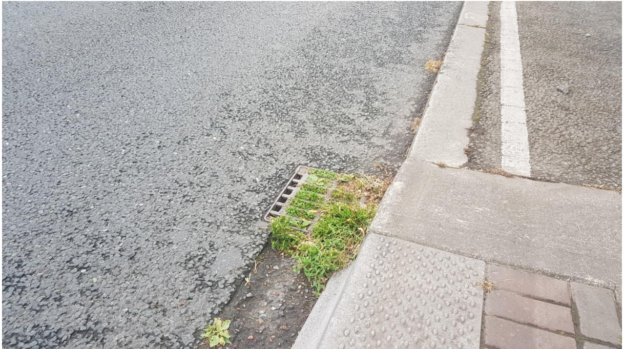
Figure 42: Blocked gully adjacent to Bus Stop on Brewery Rd N31
