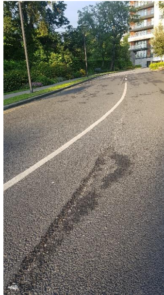
Figure 47: Existing Joints unravelling on Access Road
