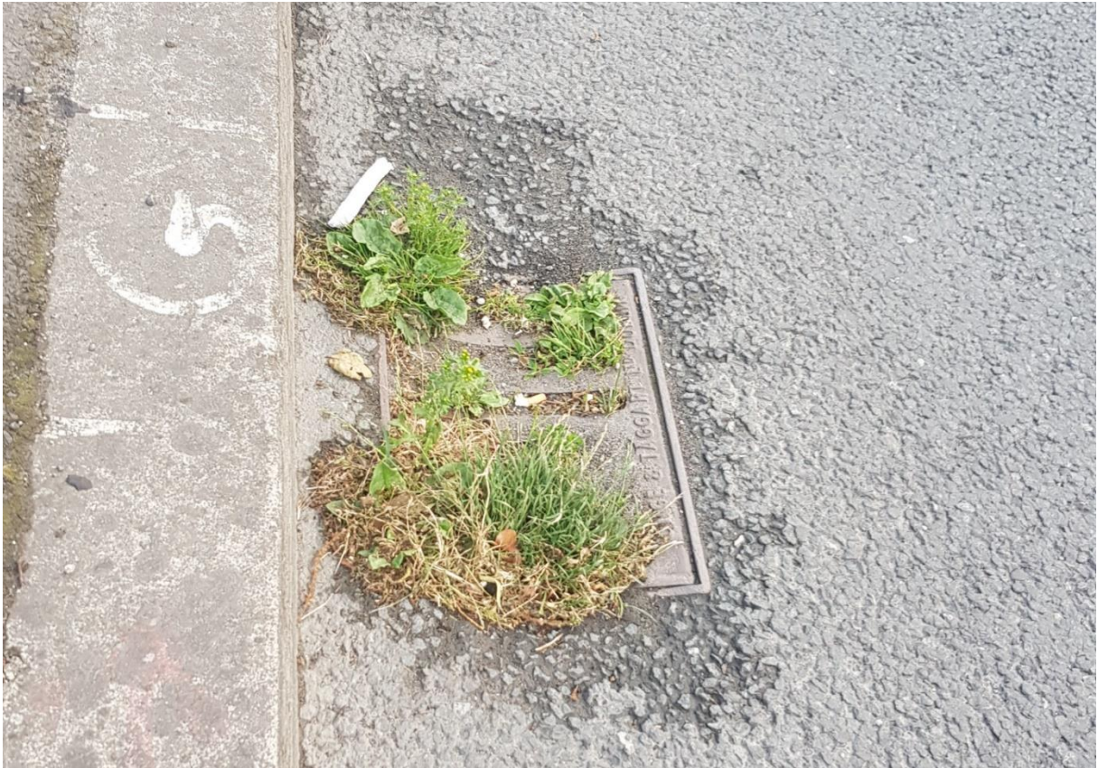
Figure 44: Blocked Gully on N31 adjacent to site
