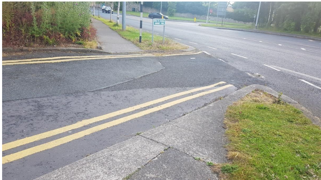
Figure 38: Tactile Paving Absent
